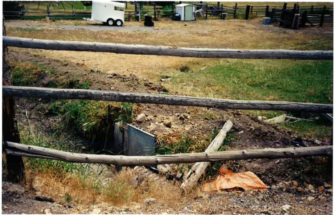
Headgate in ditch Delivery System
