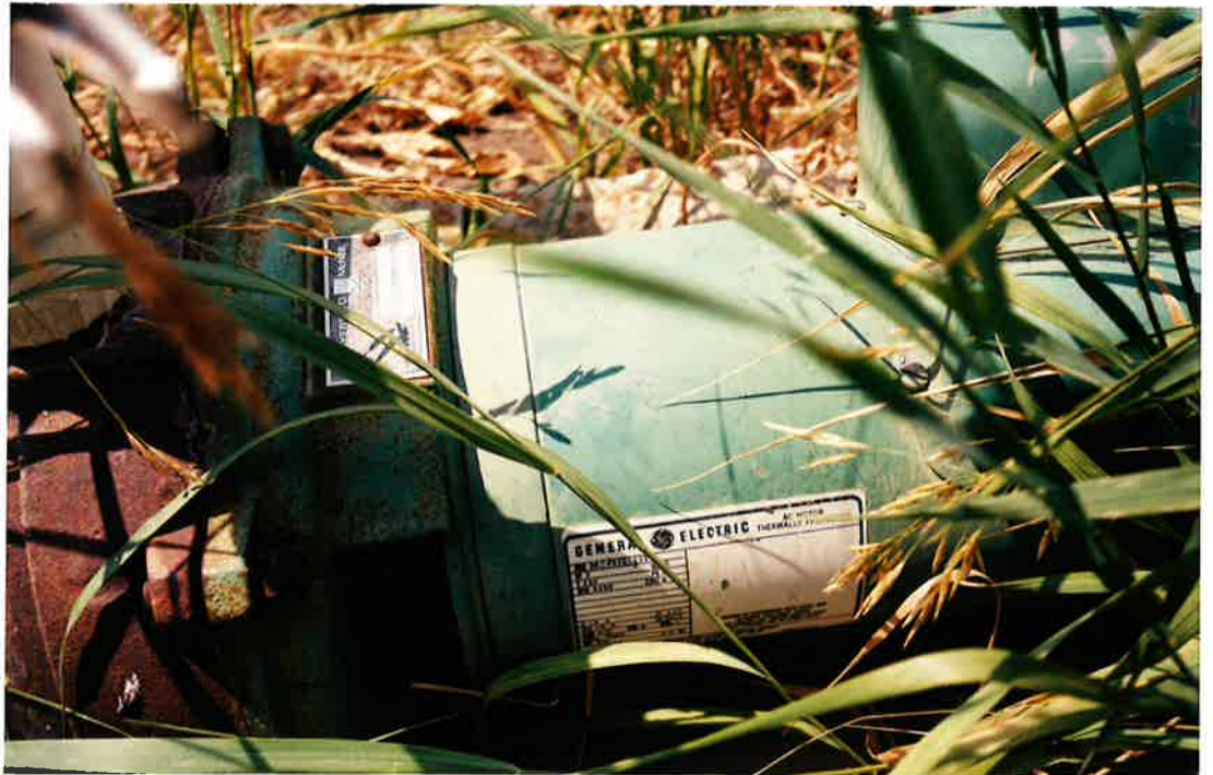
looking @ Pump. Pump info in FE Notes.
