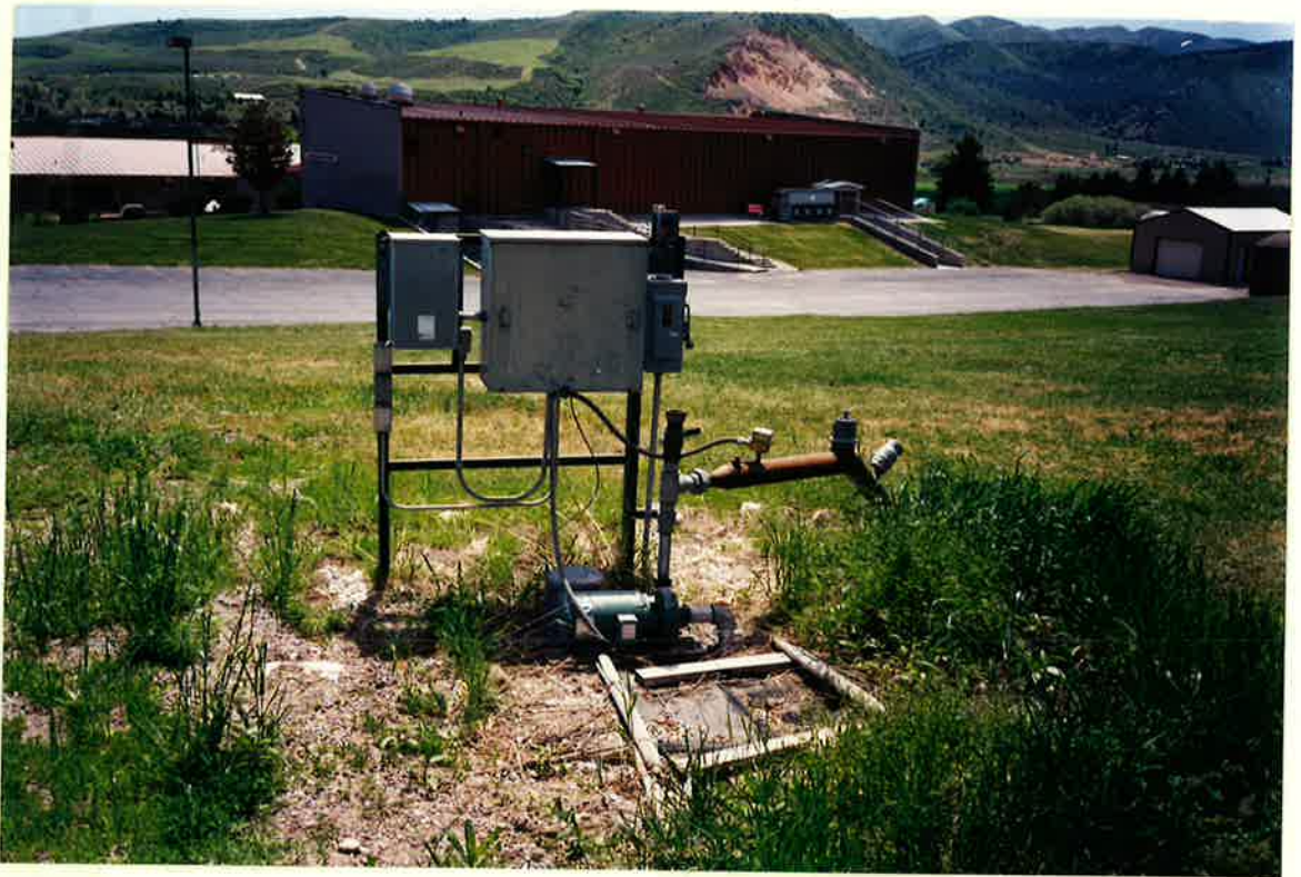
Looking S at pump where Rapid Creek Water is pumped to irrigate around the Elementary School.
