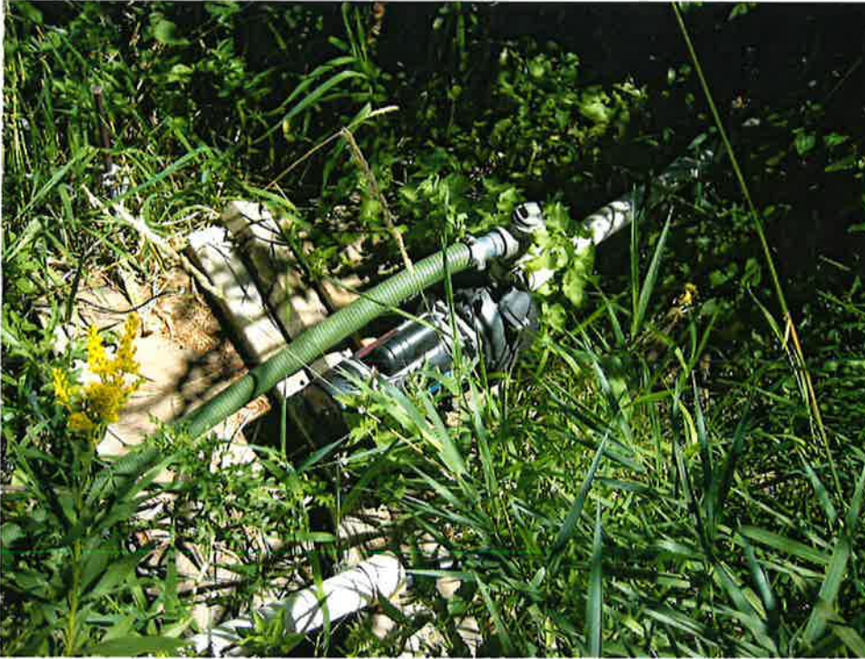
Looking at POD pump. White PVC is the intake line (csaxton).
