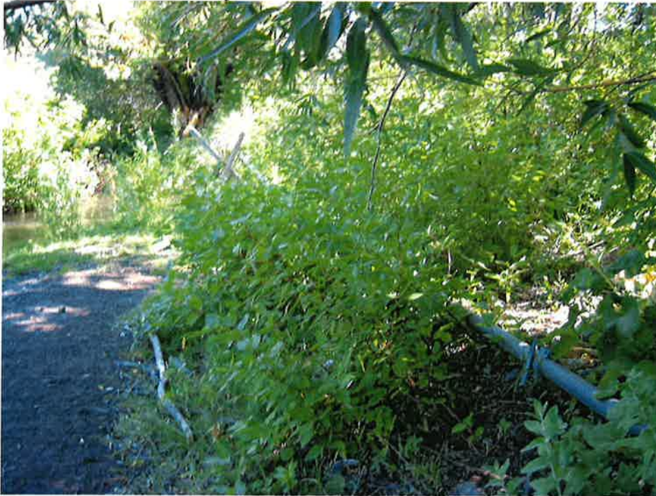
Looking South East at pipeline that supplies water to claimed POU (csaxton)
