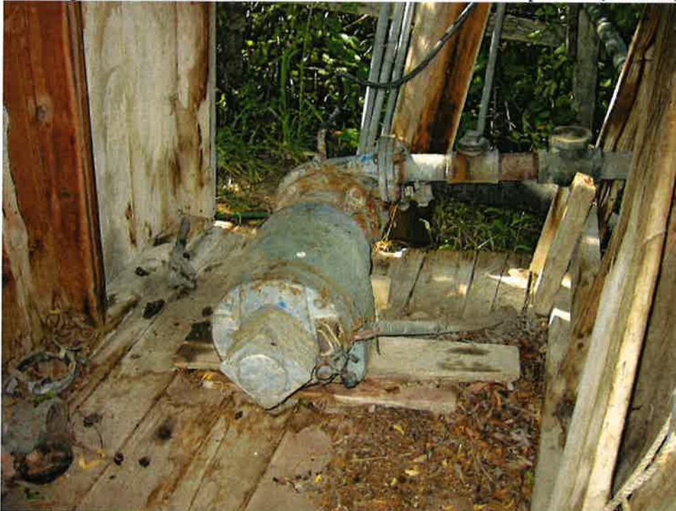
Looking South at Pump. Pump Info: Make = Jacuzzi; HP = ?; Intake = 4" line; out flow = 3" line (csaxton).
