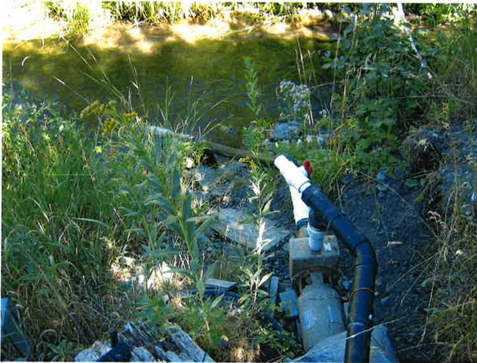
Looking East at POD pump. Pump Info: Make = Sta-Rite; HP = 5; Model = TVB184TCDR7011DNL (csaxton).
