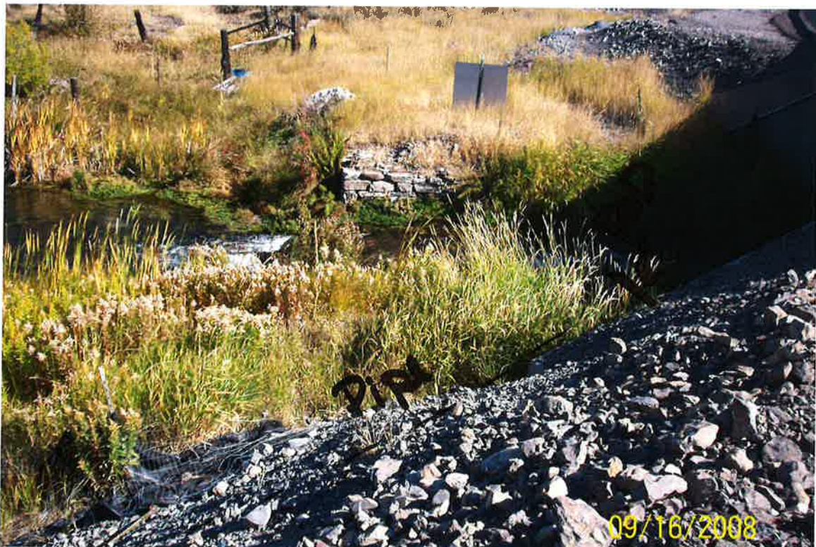
Photo 4: Shows the rock slide that crushed or collapsed pipe. Claimant plans on digging the pipe out & replacing it so he can resume irrigation.
