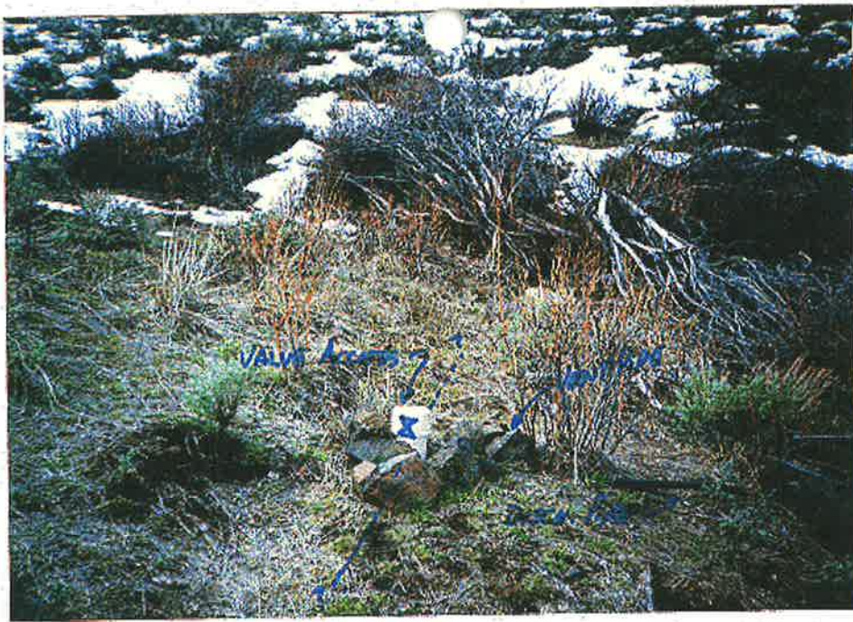
Photo 4. Looking Southwest AT BUCK SPRING(S). NOTE VALVE ACCESS PIPE (WHITE W/ CAP) & DISCHARGE PIPE (BLACK).
