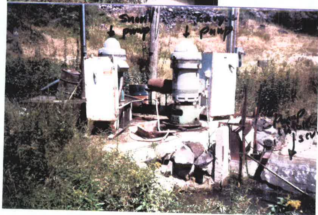
looking North East at pump arrangements
