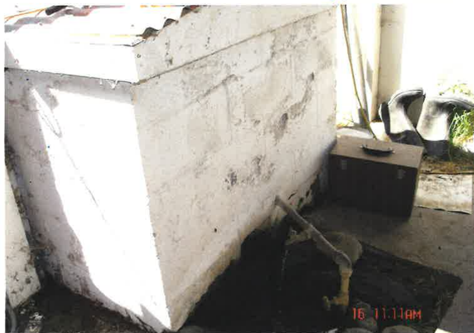
Well house Artition well 200 feet deep
