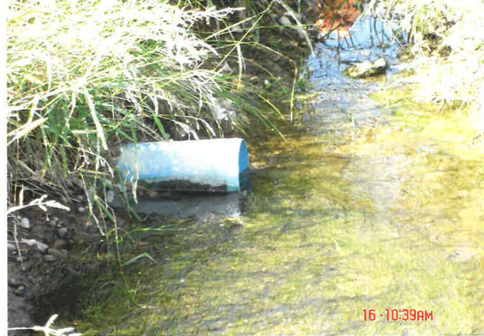
15x Pipe from head gate Across road.
