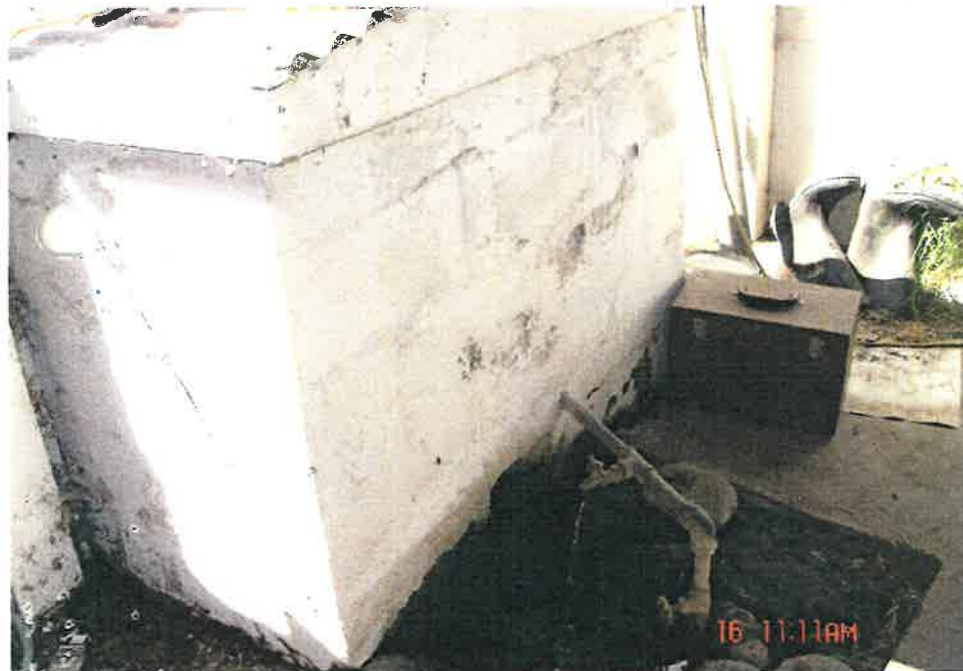
Well house Artition well 200 feet deep
