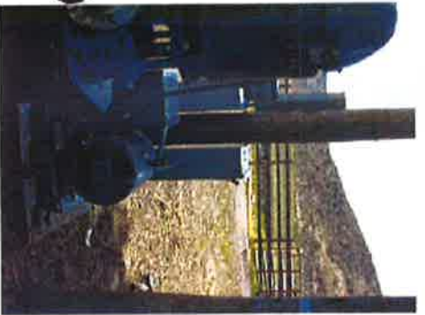
Well, Booster Pump, and GPS Tag A0004195
