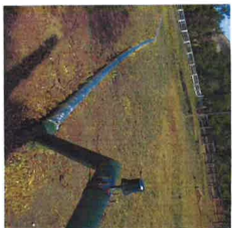
McCrometer Flow Meter 8" main line, buried to pivot
