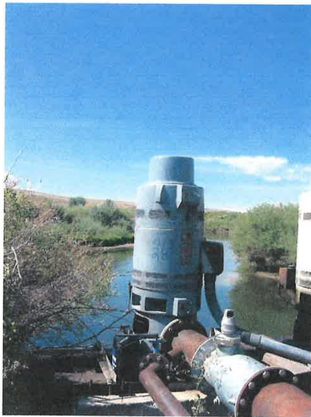
200 HP River Pump (Blackfoot River)
