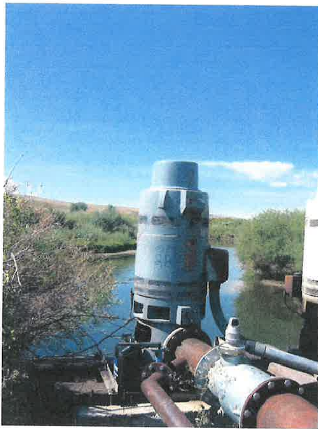
200 HP River Pump (Blackfoot River)
