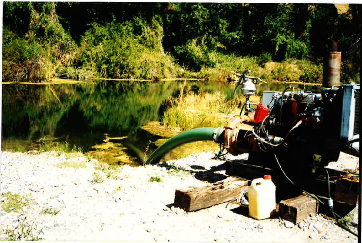
A. 23 11210 P.O.D. 140 H.P. SN# 774098 DETROIT DIESEL 4 CYLINDER ENGINE TAG# A.0012439 6" INTAKE LINE 6" MAIN LINE.
