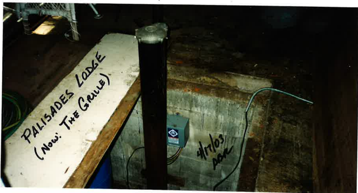
SHOWS CASING INSIDE BLOCK WELL HOUSE.
