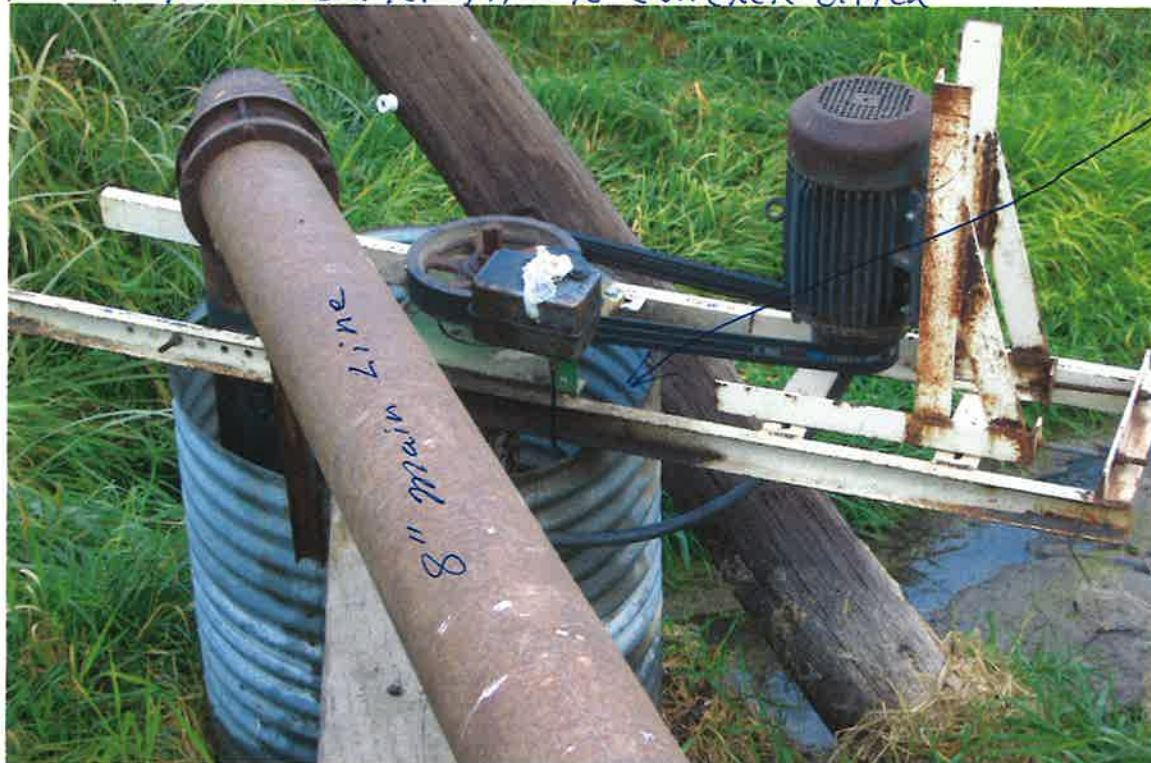
PRC#1 pump + outlet pipe to concrete ditch
