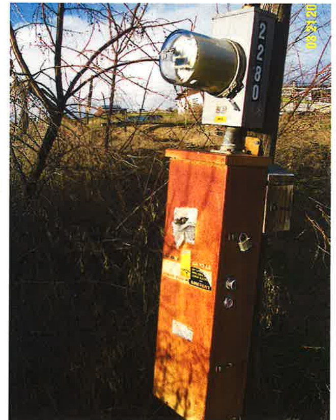
Armenta Meter & Panel
