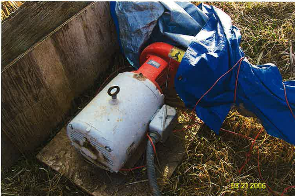
Armenta Pump 20 HP Centrifugal
