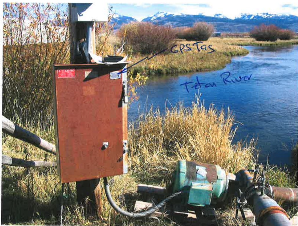
A22-00587 - Relift pump (redirection)
