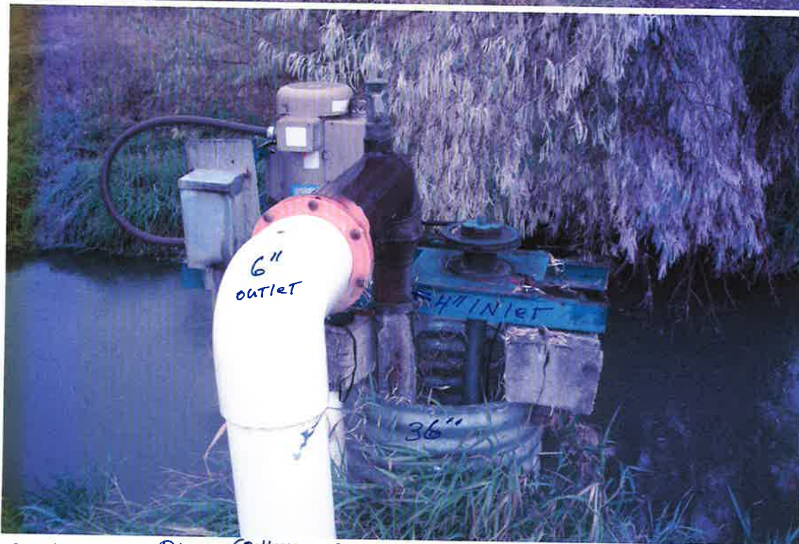
PIC#2 Pump(3HSP) Baldor motor
