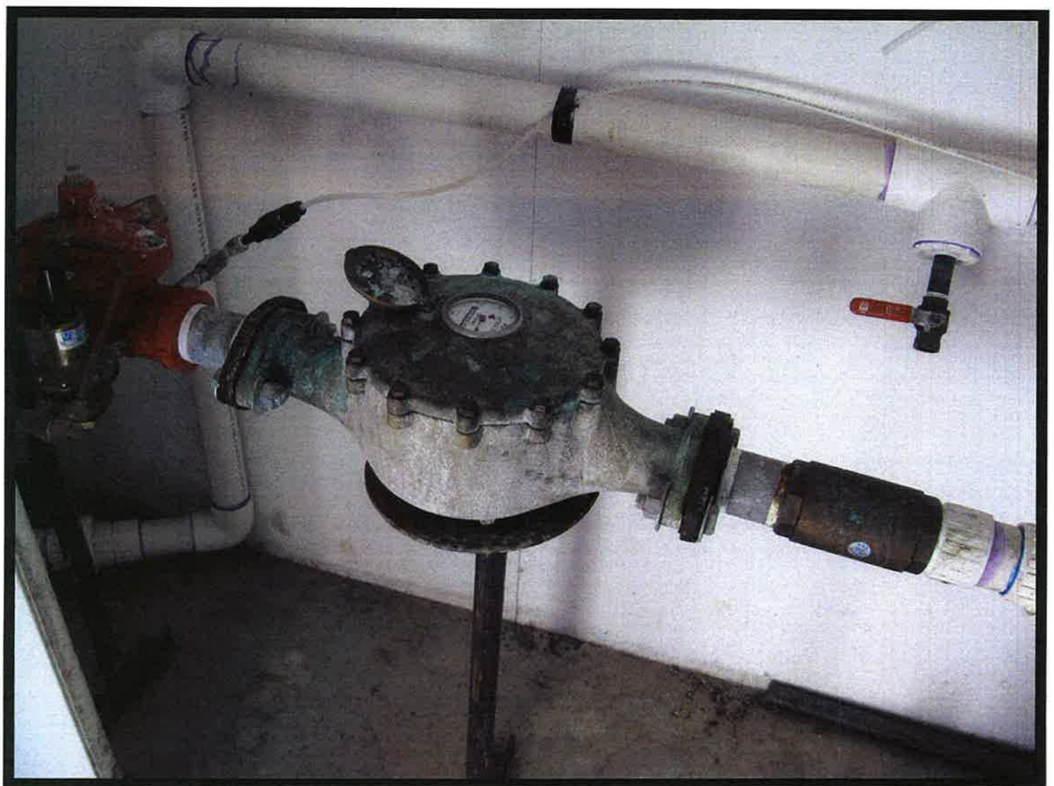
Friends Well In-line Flowmeter
