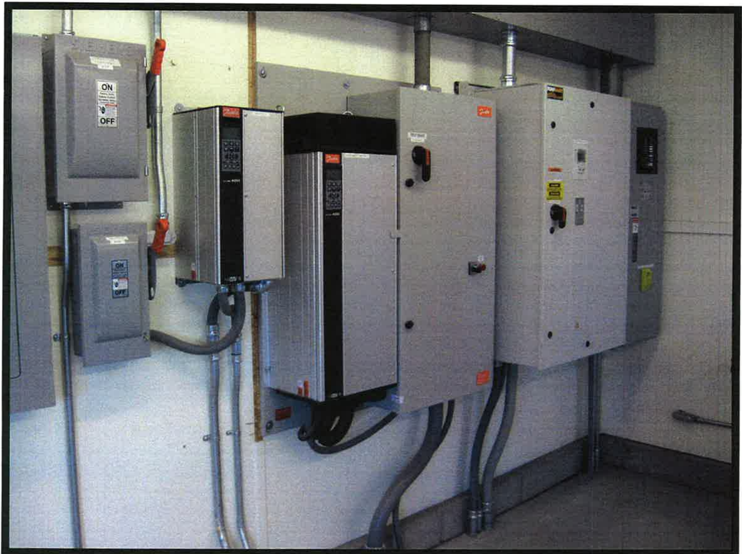
Butler Well Pump System Controlling Works
