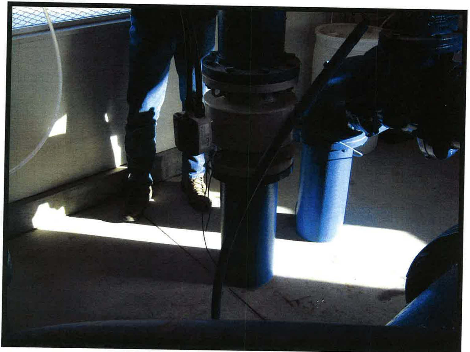
Butler Well In-line Flowmeter
