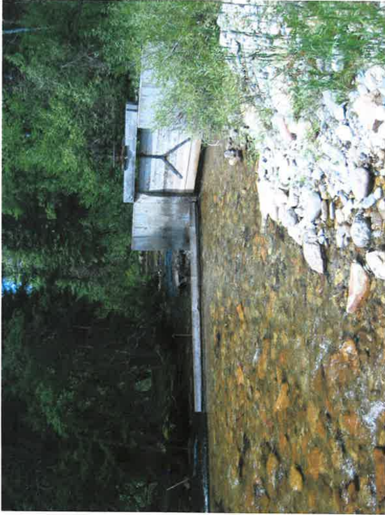
Garden Irrigation System (Starkey Creek) Hill Canal headgate in Wyoming
