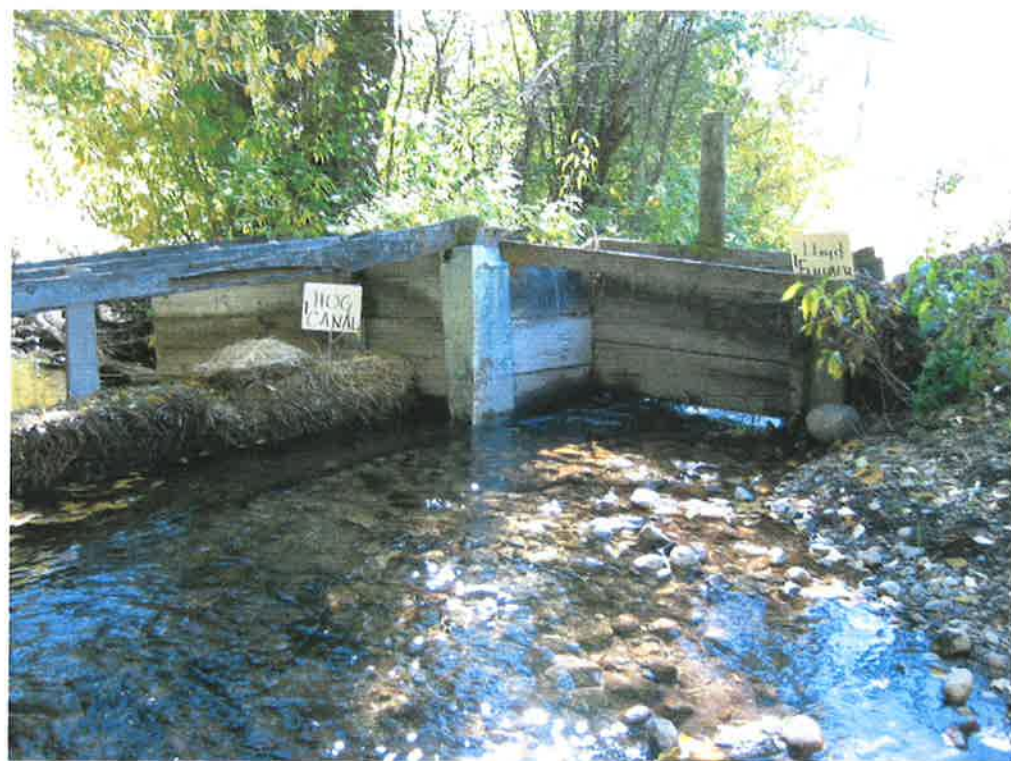
Lloyd Fullerton's Headgate over Hog Canal. Wyoming 5106. Diverts to Private Ditch
