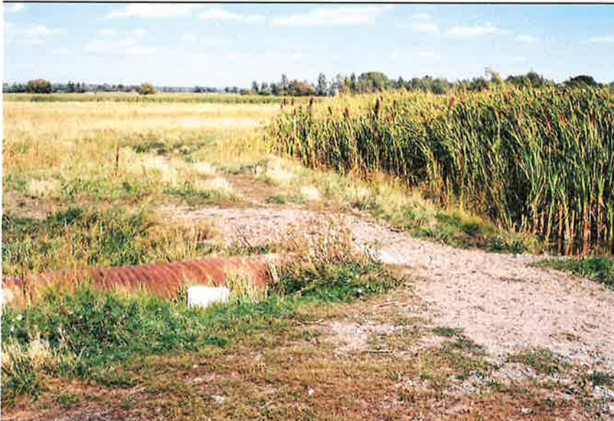
First point of diversion. Water flows from right to left. Culvert is blocked to back up water causing sub-irrigation of pastures. Similar pattern of use for all other PODs shown below.
