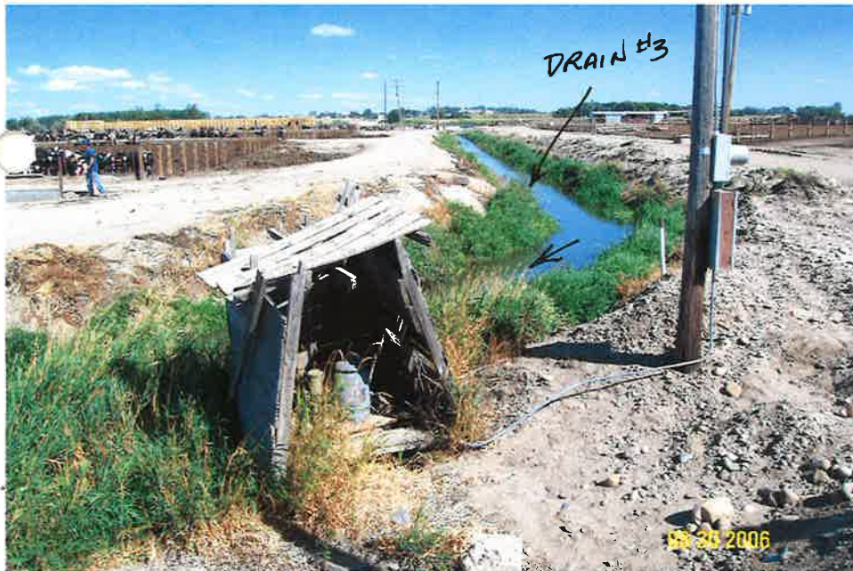
LIFT PUMP LOOKING EAST PQU. WEST PUMPLINE TO DITCHES
