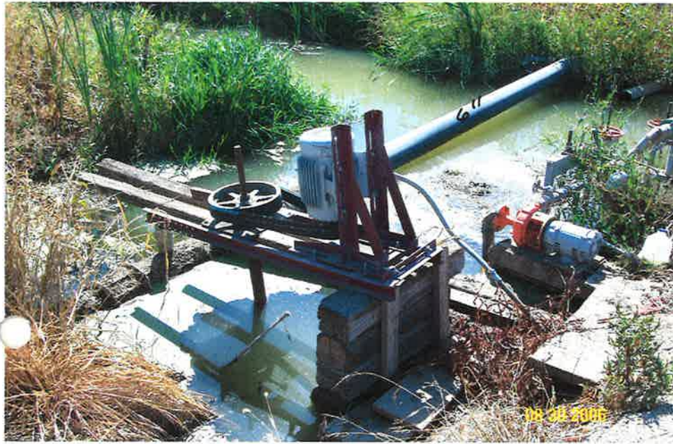
PUMPING PLANT PUMPING FROM DRAIN #3
