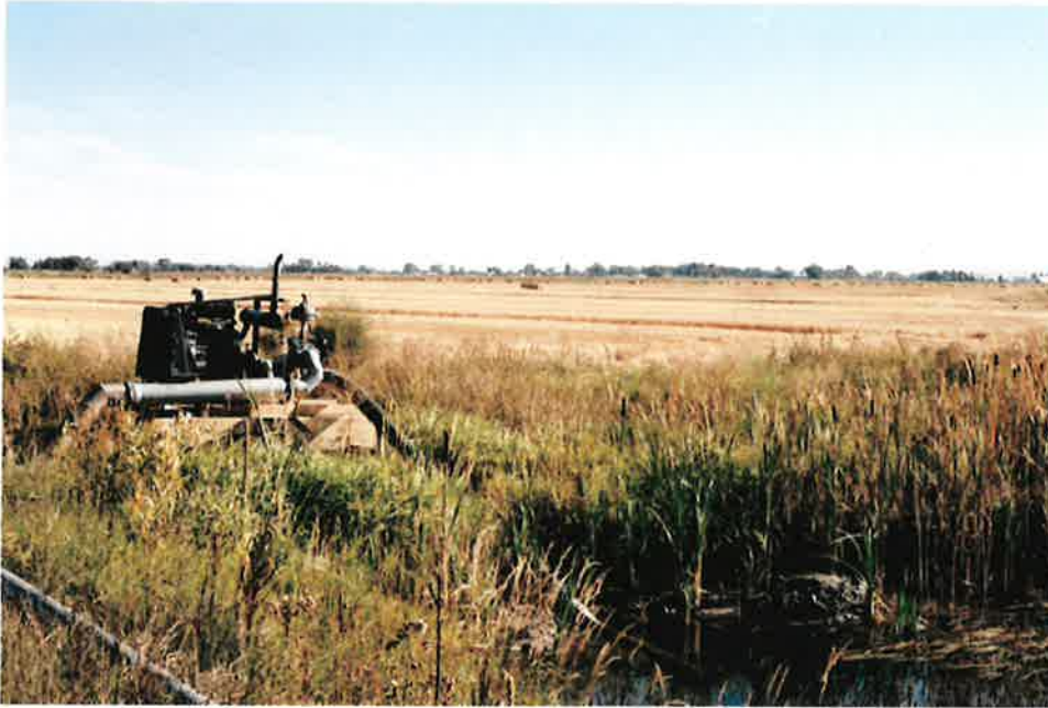
Photo #3. This is the pump that can be used for this water right. This photo was taken at the location of POD for A22-10933.
