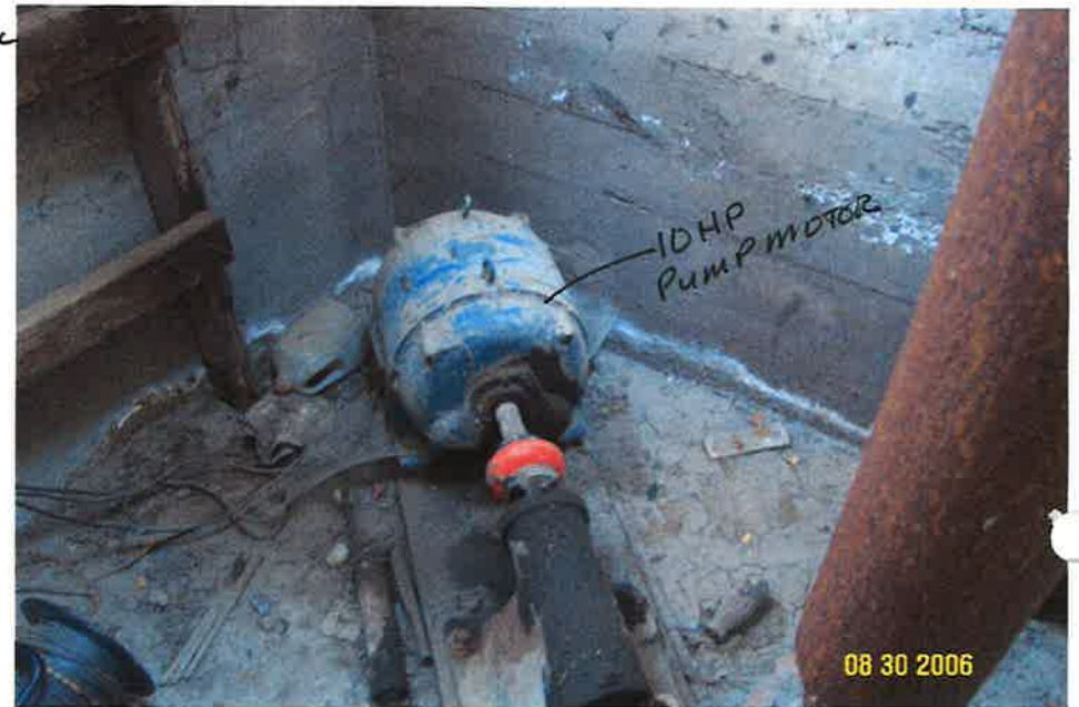
63-5230 WELL PUMP BY HOUSE
