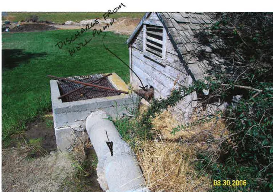
WATER IS DISCHARGED INTO THIS BOX FROM PUMP FLOW GOES INTO MAINLINE ALONG ROAD
