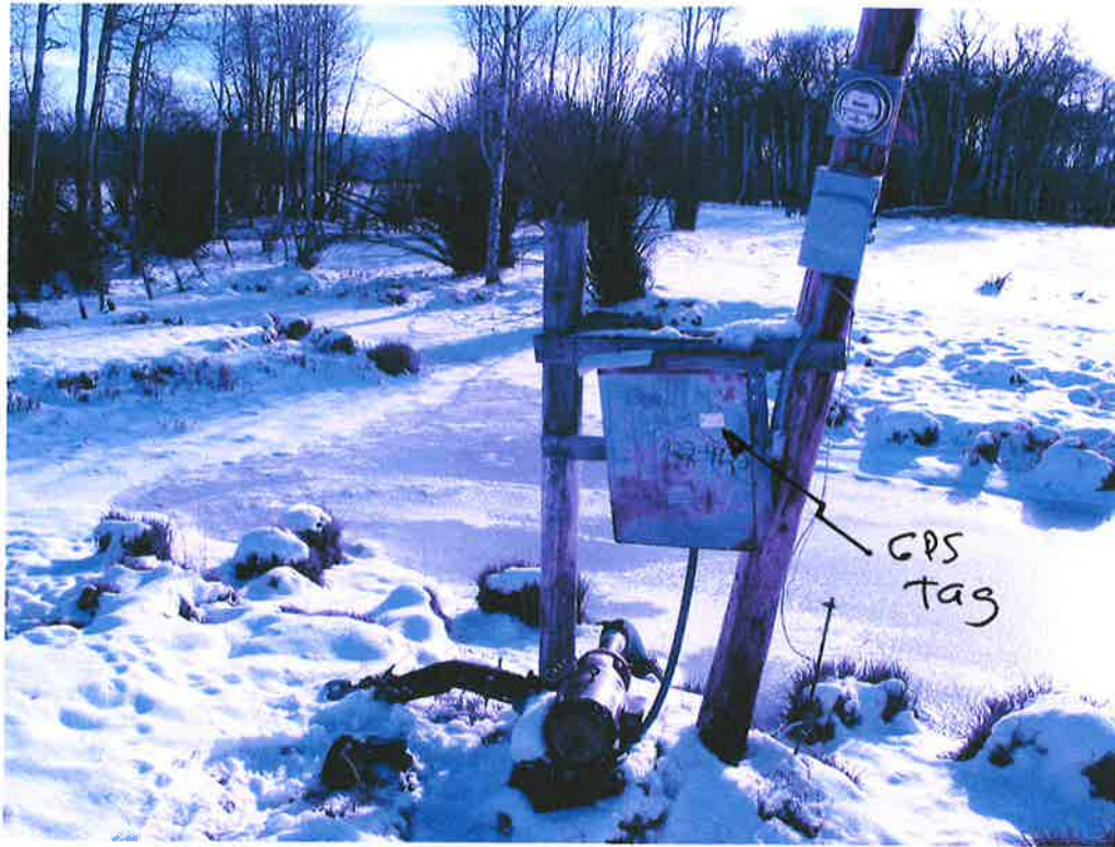
A22-4123 - pump at spring
