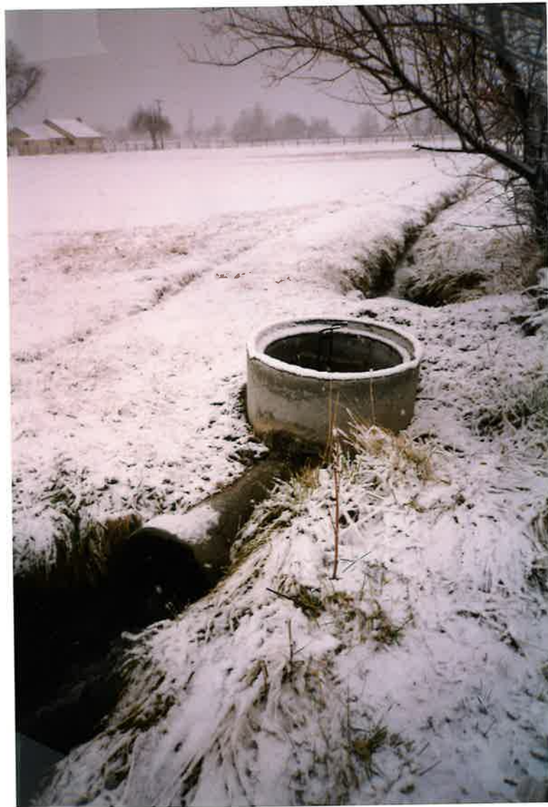
Riser at end of pipeline from SANDS ditch.
