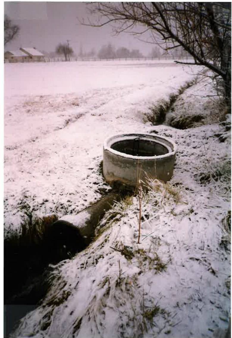
Riser at end of pipeline from SANDS Ditch.
