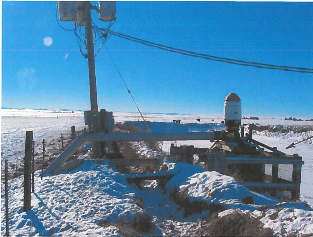
North Relift pump in pond to mainline
