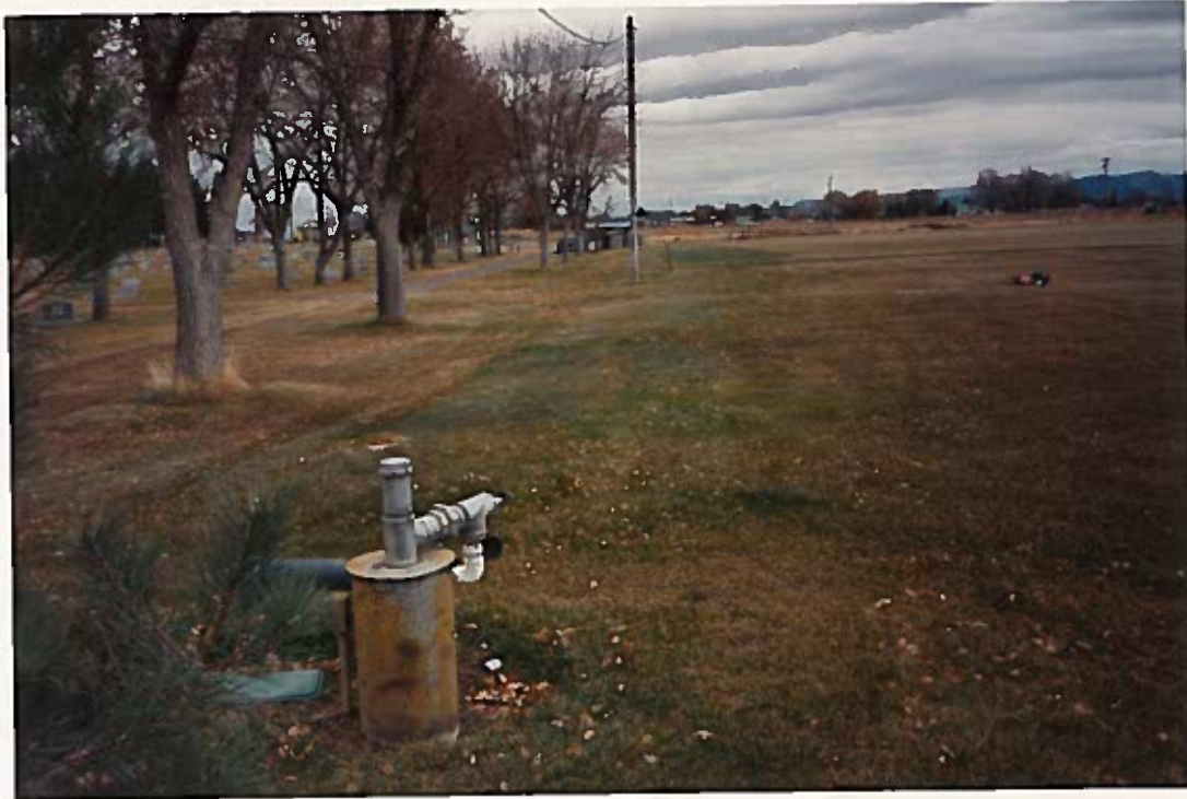
* Facing East. Point of diversion at west end of the cemetery. Submersible motor and pump.
