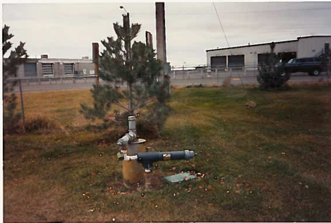
* Facing west. Point of diversion at the west end of the cemetery. Submersible motor + pump.
