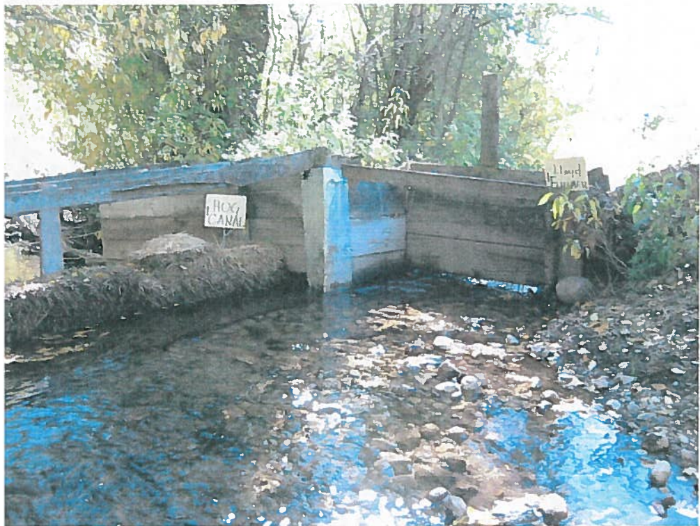
Lloyd Fullumon's Headgate over Hog Canal. Wyoming 5105. Diverts to Private Ditch
