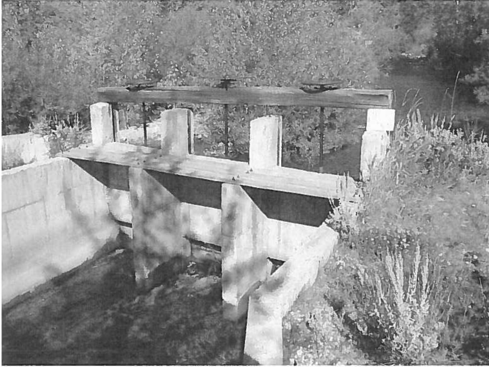
HOG CANAL DIVERSION (WYOMING SIDE) OFF SO LETCH CK ALSO SERVES LLOYD FULLMER
