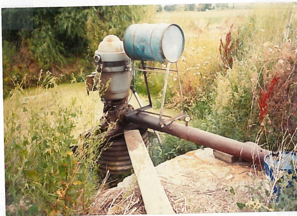
Pump in Diversion from Buckeye Ditch
