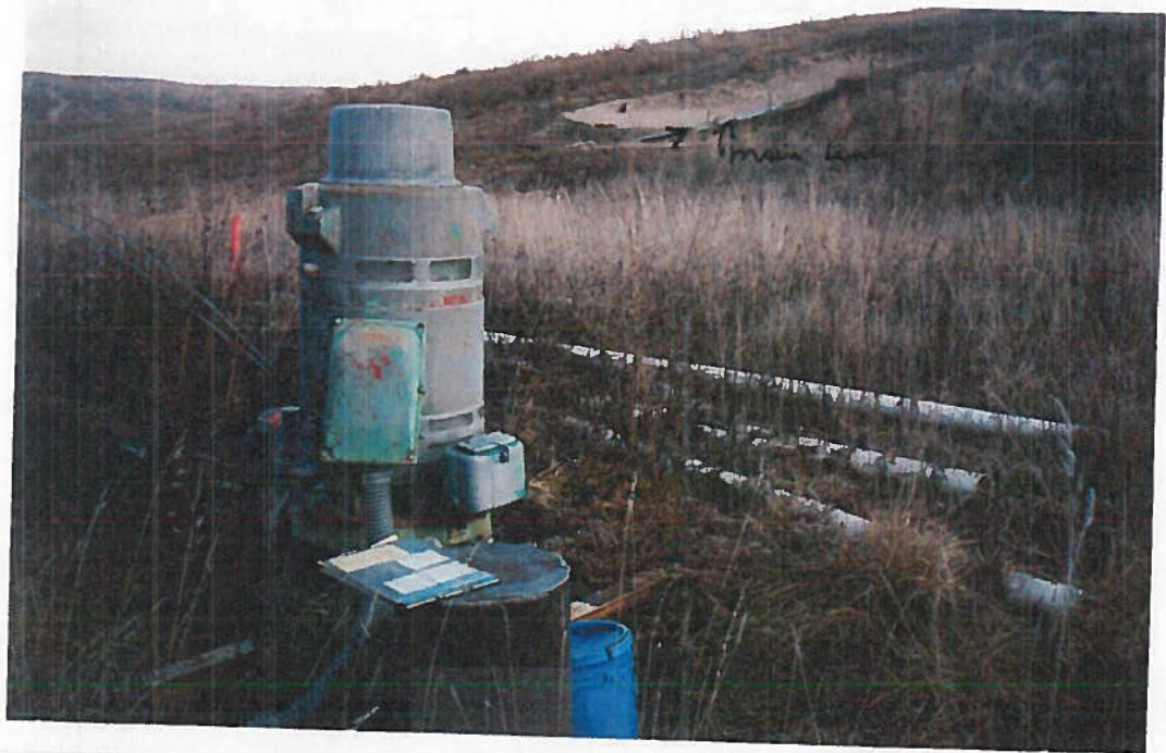
PHOTO THREE- View northeast of well No. 2, located in NWSW Sec. 1. 10" main line from pump, and 8" main line up hill.
