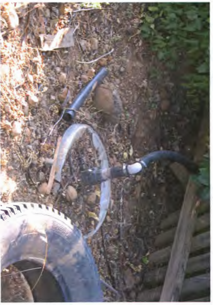
water pipes on property
