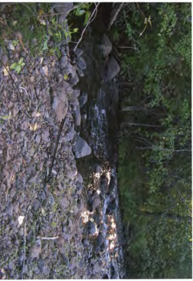
POD - Due to the high water years the diversion has been filled w/ rock + debris -
