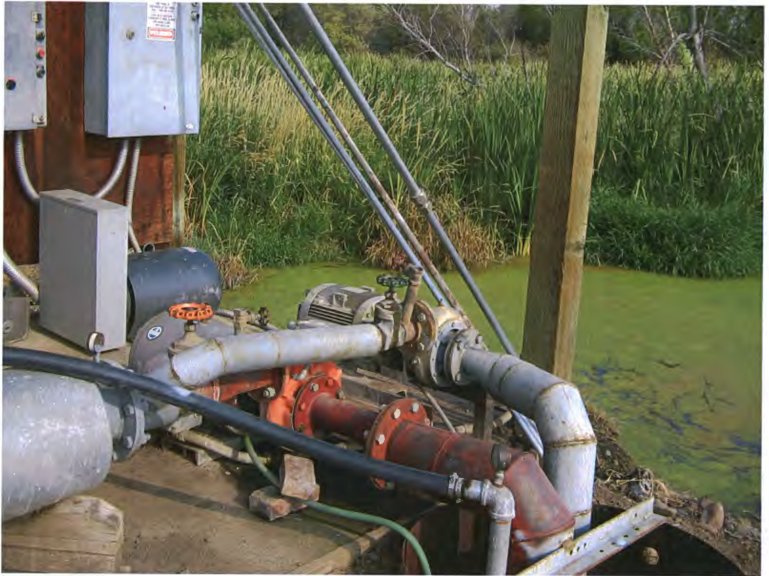
Pumps for 67-4072 8/16/06 Exam
