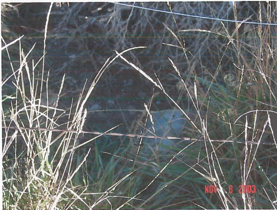
Culvert that takes waste water from POD #2 under road onto property.
