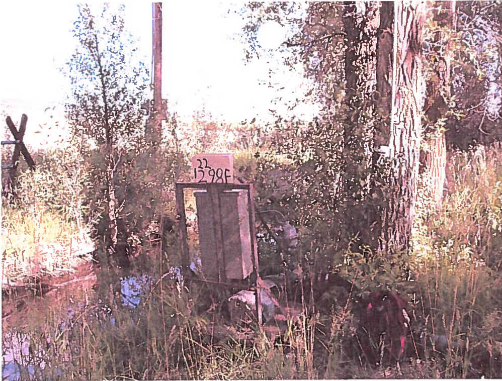
Tom Knight pump on Horseshoe Creek. Tag on electric panel.
