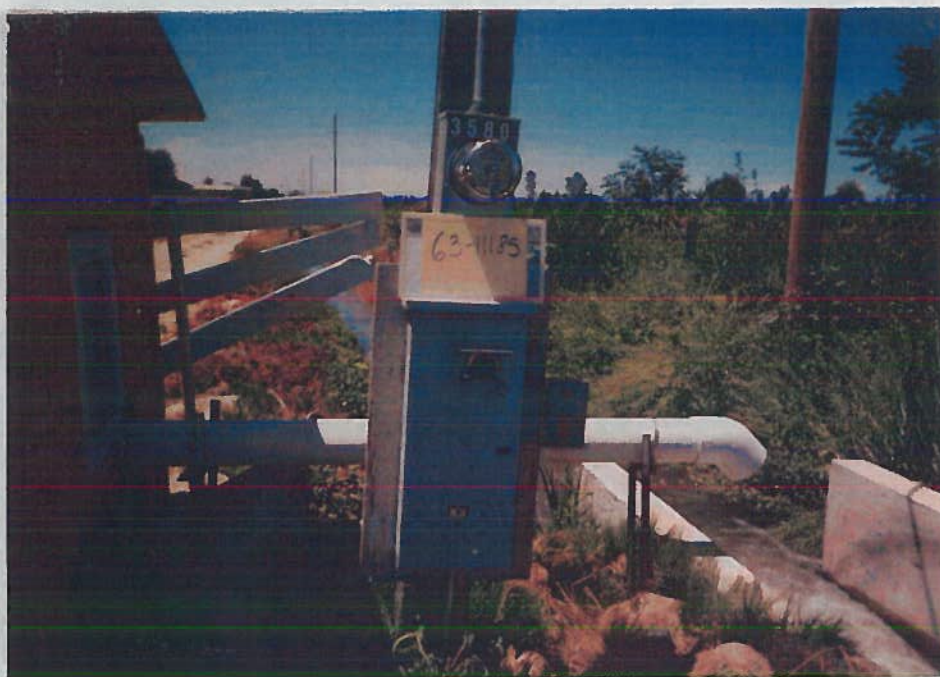
pump control box
