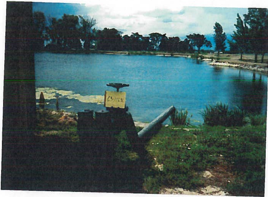
Picture of well + pump with a 6" open discharge line into holding pond. Picture taken looking south.
