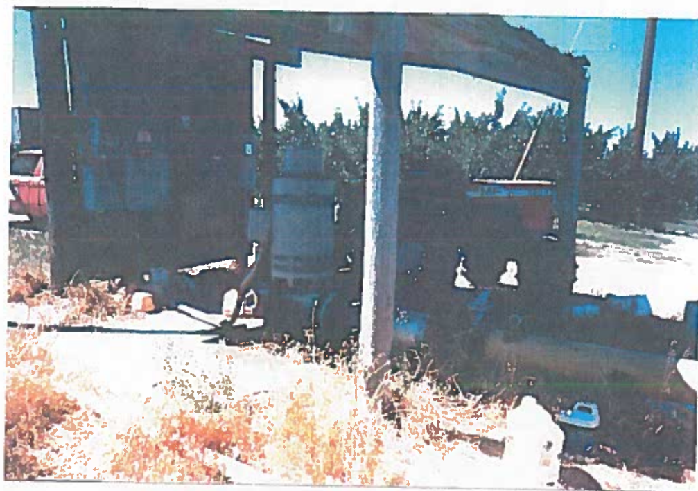
Pump for Permit 63-9818 New well #2
