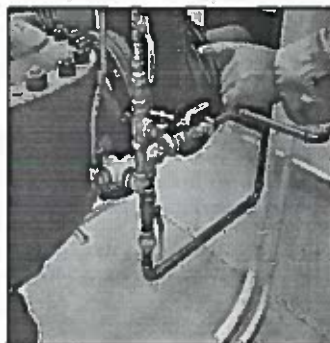
Fig 9 – copper cooling piping
