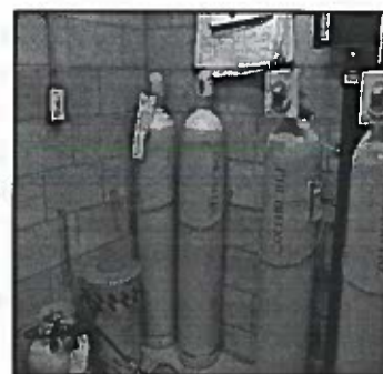
Fig 6 – Chlorination room associated with the 500,000 storage tank.
