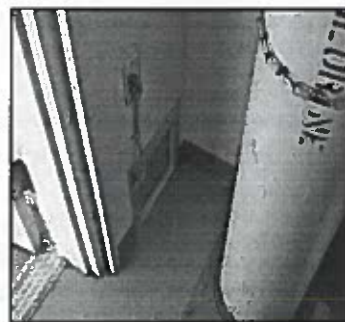
Fig. 6a – Chlorination room associated with the 1 mg. storage tank.
