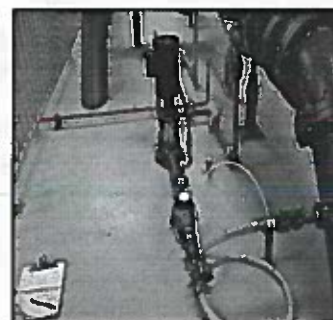
Fig. 8 – Chlorine injection site booster pump.
