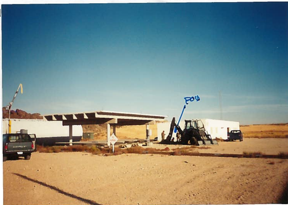
Photo #2 Looking NW from the NESW Sec 33 10-1-96 Showing the POD & POW - Natl Guard Personnel are installing a flow metering device. MPRCH Facility
