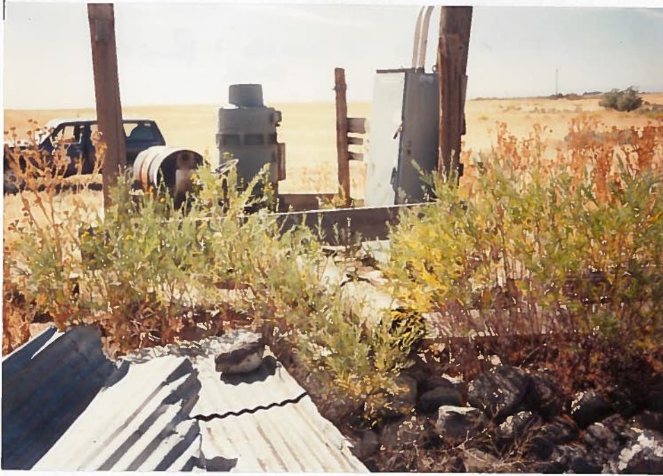
Photo #6 Looking N.E. From NW corner of 4S 7E Sec 16 showing well/pump #1
