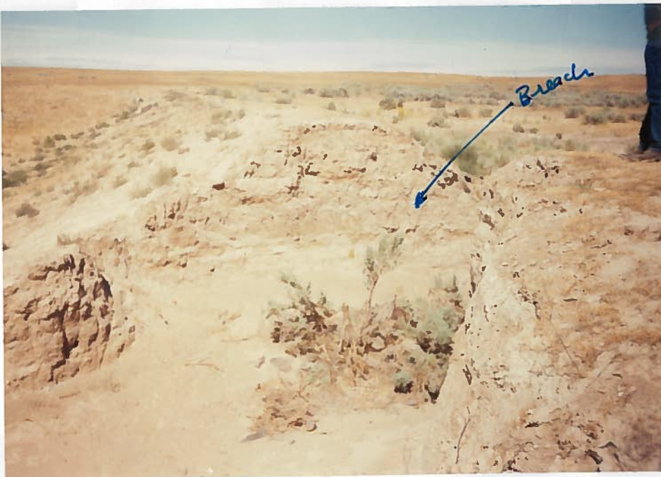
LOOKING NW FROM 45 7E Sec 4 NW 1/4 at the Break in the Dam Photo #9
