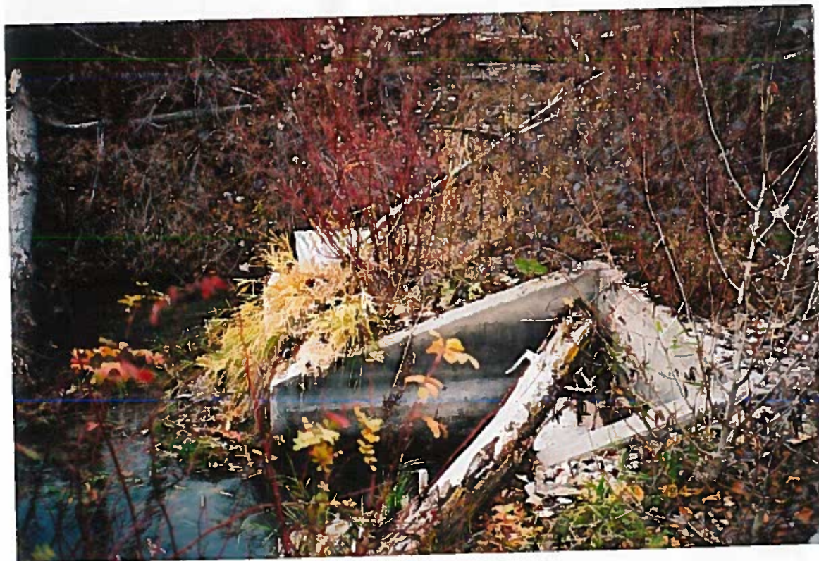
A22-653A flapper gate @ discharge end of return culvert. photo # 4 on map
