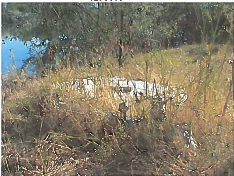
Old POD (not presently used). Pipe shown is terminated.
