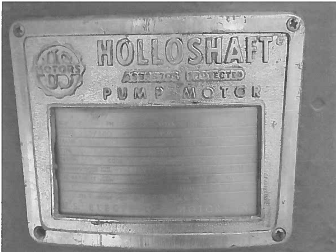
Pump #2 (Short Coupled Turbine Pump, Data not available)
