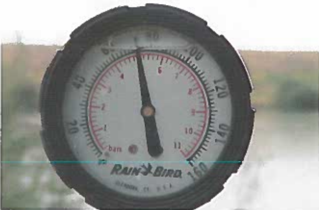
Pressure at pump.
