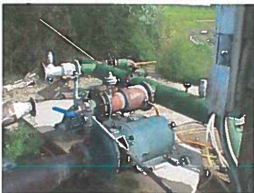
Main Motor and pump at POD.
